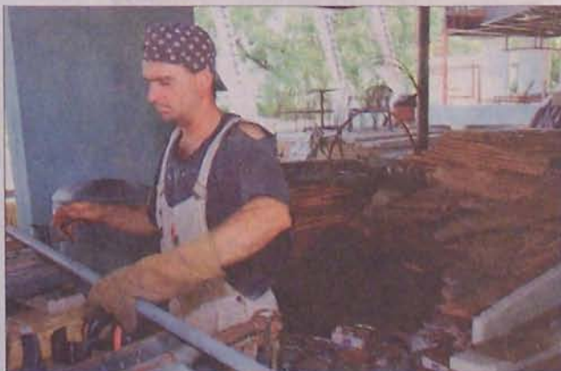
Architect Michael Calvino cuts galvanized steel pipes for a balcony rail. Behind him are planks of eucalyptus, which he cut by hand from a fallen tree.
