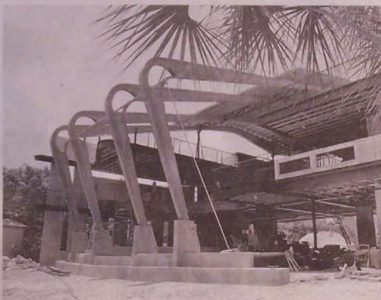
The house being built on the Little Manatee River in Ruskin for Stanley and Sharon Woodruff features hanging walls, dyed concrete floors and a soaring price tag.
