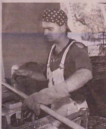
Architect Michael Calvino works on cutting pipes to size. This is the first home the young architect has built.
