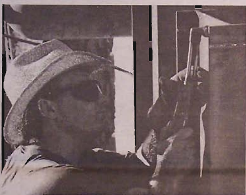
Calvino cuts a steel beam for the roof of the Woodruff home in Ruskin.
