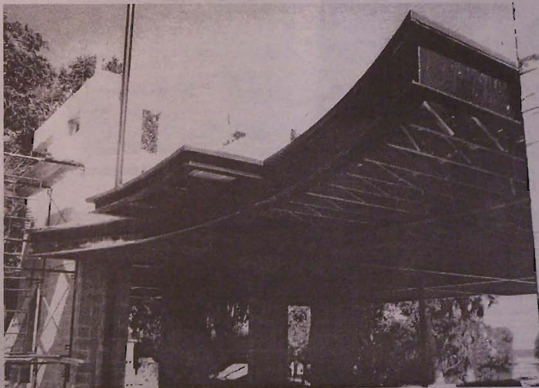
The house Mike Calvino is building in Ruskin was designed to take advantage of prevailing winds and a magnificent Gulf view.
